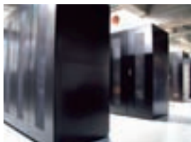
Data center operating in the ICT outsourcing field
